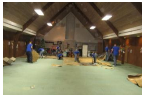
CHAPTER 872 CONTINUED ITS SUPPORT OF THE MISSION CONTINUES BY RIPPING UP AND REMOVED CARPET AND PAINTING CLASSROOMS FOR THE COMMUNITY LINK ORGANIZATION.
